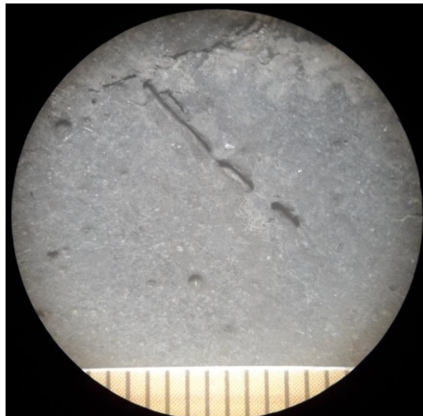
Fig. 6. (b) Melting of PP fibres in polymer fibre concrete at high temperature (400oC).
