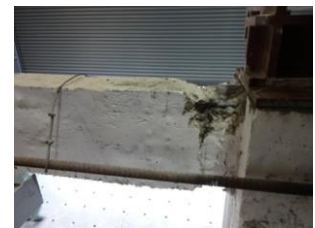
c) Crack at the right beam
