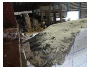
b) Crack at the left beam
