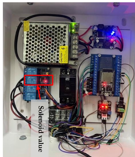
Fig. 15. Relay operate to initiate solenoid for feed distribution to the pond.
