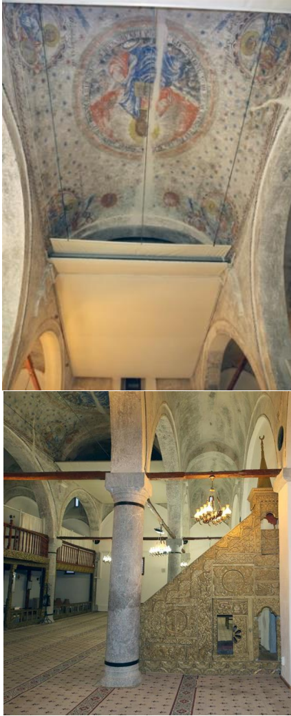
Fig. 2. a) The frescoes in the vault b) The cracks formed after the earthquake.
