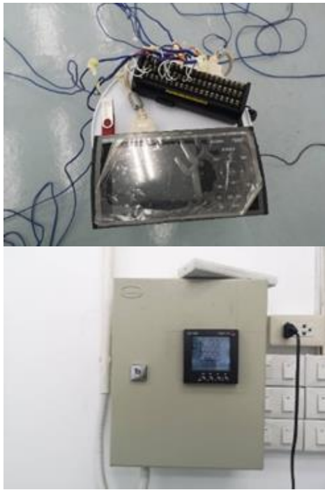
Fig. 2. Data logger and energy meter.
