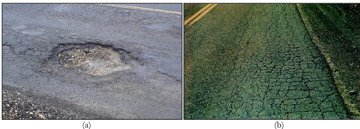
Fig. 2. Deteriorated pavements due to Water induced damage, (a) pothole (b) alligator cracking [2].
