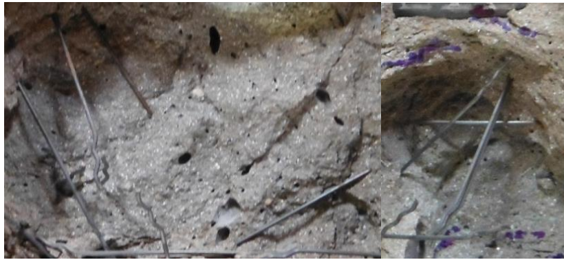
Fig. 14. COL-B: Hook end embedment in spalled-off concrete.
